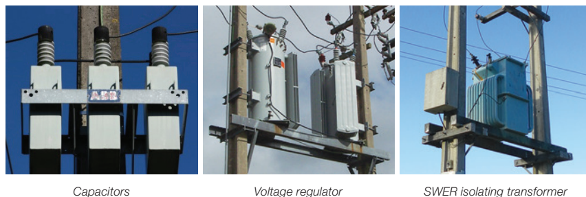
Figure 18.11: Collection of 'other' distribution transformers
