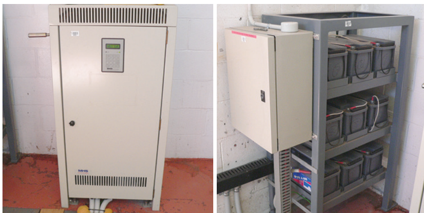
Figure 20.6: DC charger and battery bank
