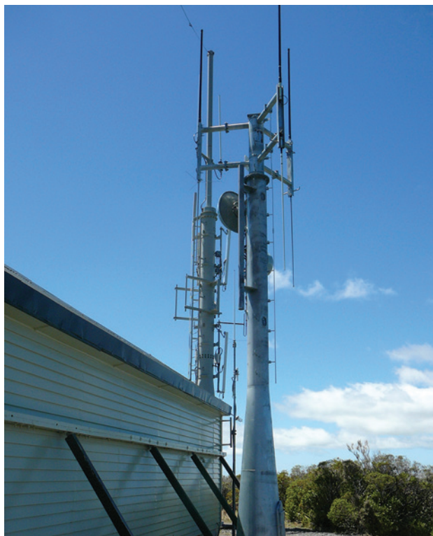
Figure 20.2: Communications mast with associated radio antennae
