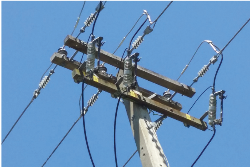
Figure 19.6: Pole mounted drop out fuse
