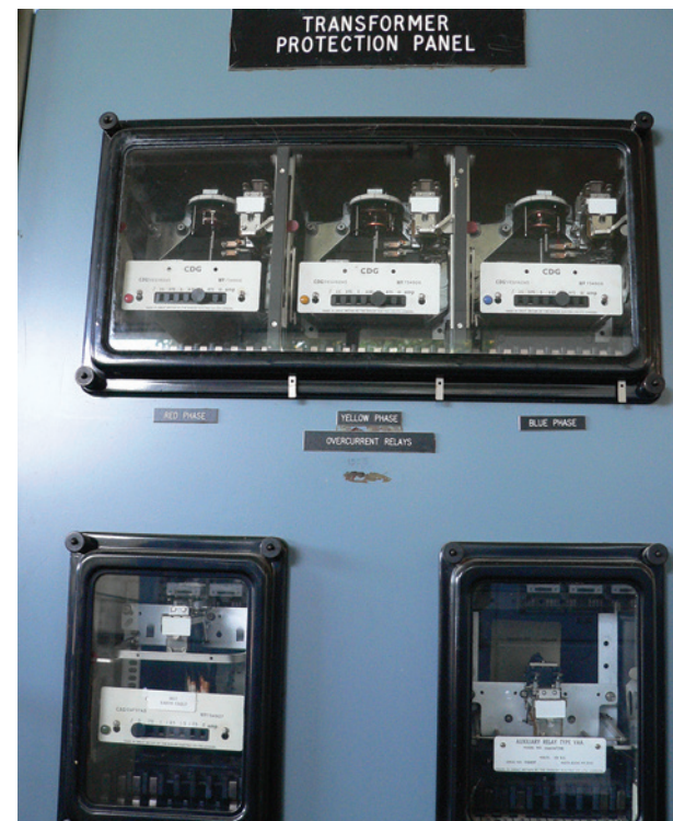
Figure 20.3: Electromechanical relays providing transformer protection
