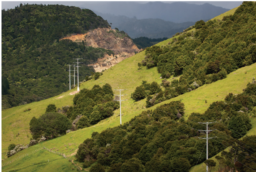
Figure 15.1: 66kV subtransmission overhead line in the Coromandel
