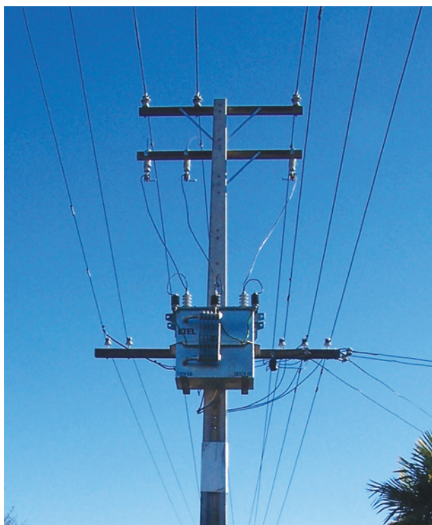
Figure 18.1: 100kVA pole mounted transformer
