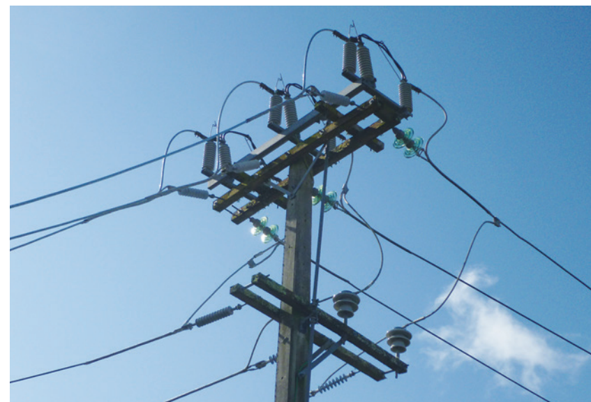
Figure 19.11: Air break switch
