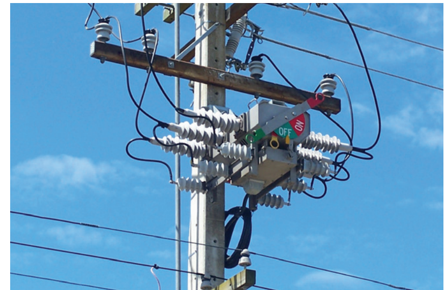
Figure 19.15: A pole mounted recloser
