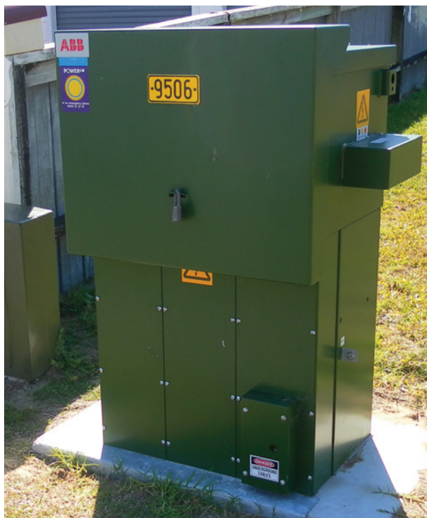
Figure 19.1: Ground mounted switchgear
