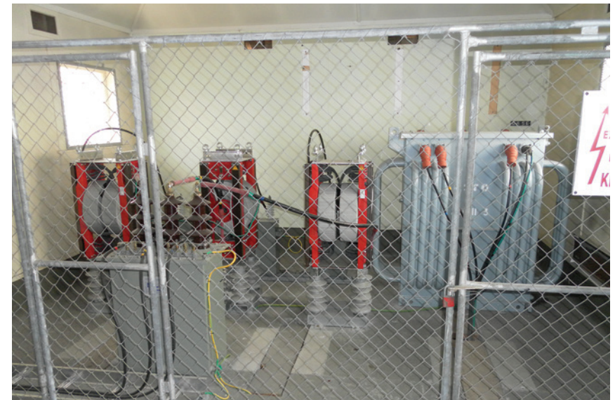
Figure 17.16: Load control injection plant
