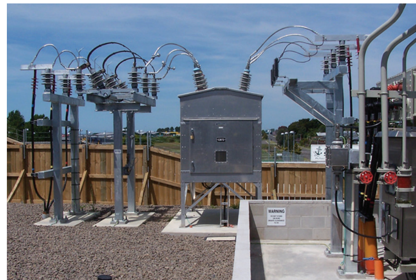
Figure 17.9: Typical outdoor 33kV switchgear bay
