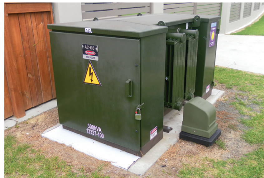
Figure 18.6: 300 kVA ground mounted transformer
