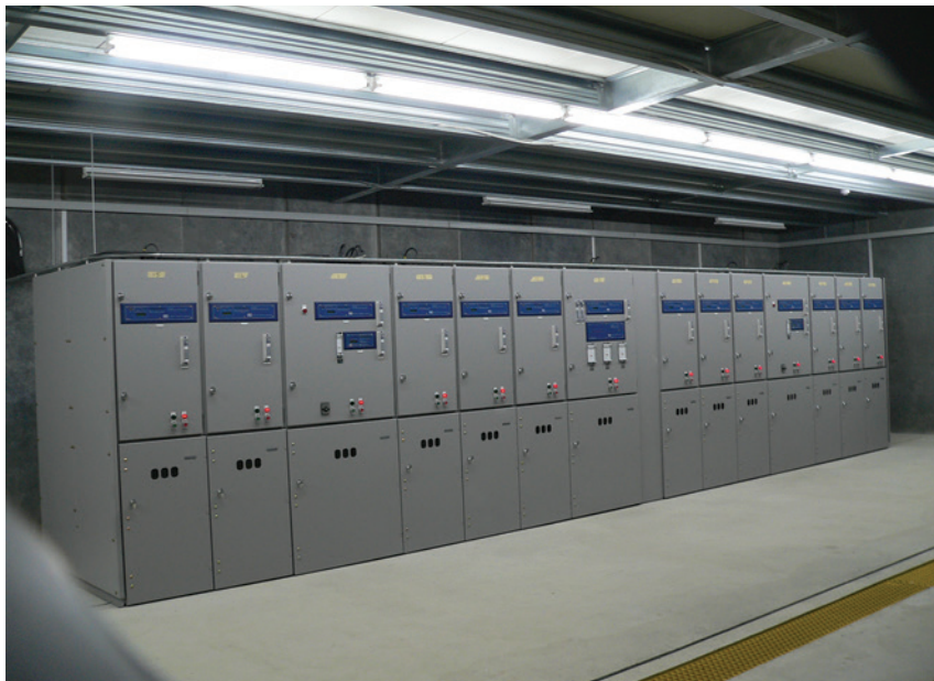
Figure 17.5: 11kV indoor switchboard at Main St, Palmerston North
