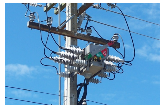
Figure 20.15: A pole mounted recloser
