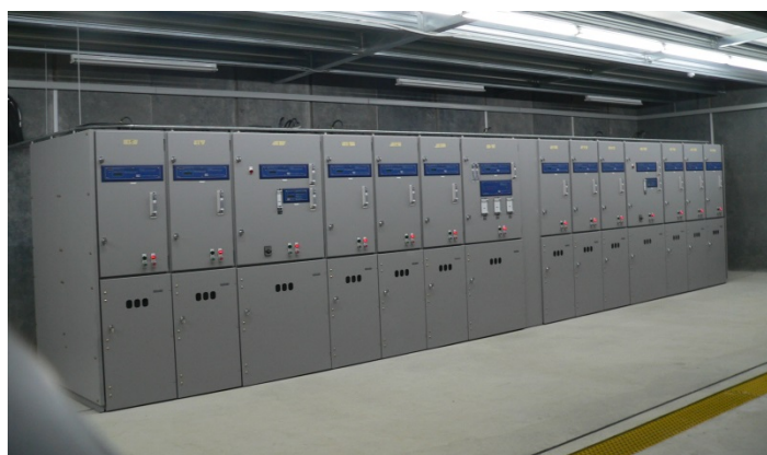
Figure 18.5: 11kV indoor switchboard at Main St, Palmerston North
