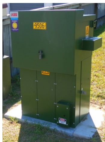
Figure 20.1: Ground mounted switchgear
