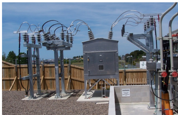
Figure 18.9: Typical outdoor 33kV switchgear bay
