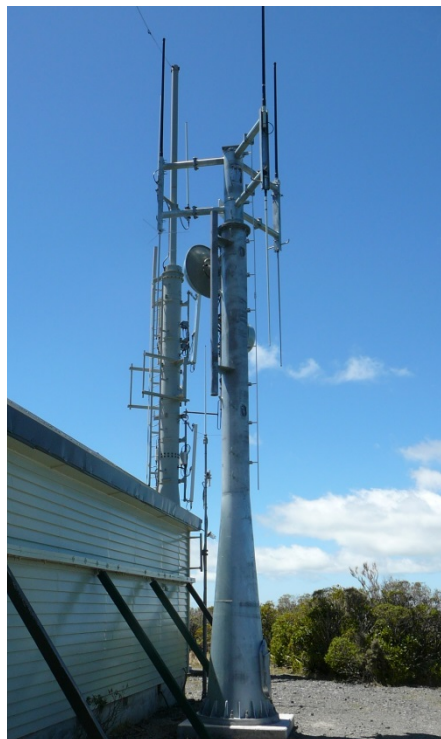
Figure 21.2: Communications mast with associated radio antennae
