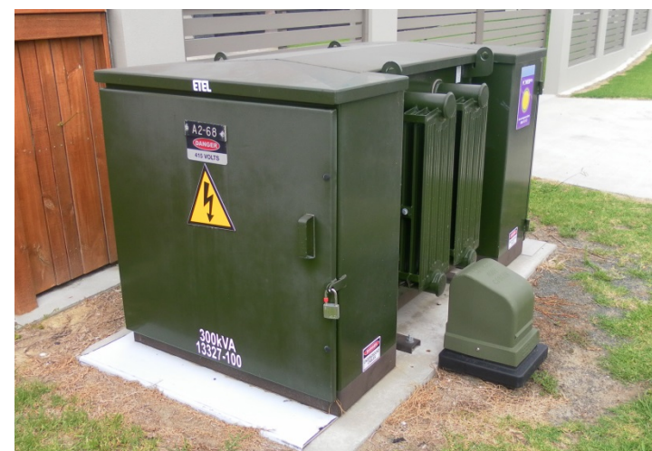
Figure 19.6: 300 kVA ground mounted transformer
