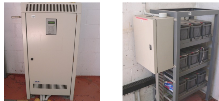
Figure 21.6: DC charger and battery bank
