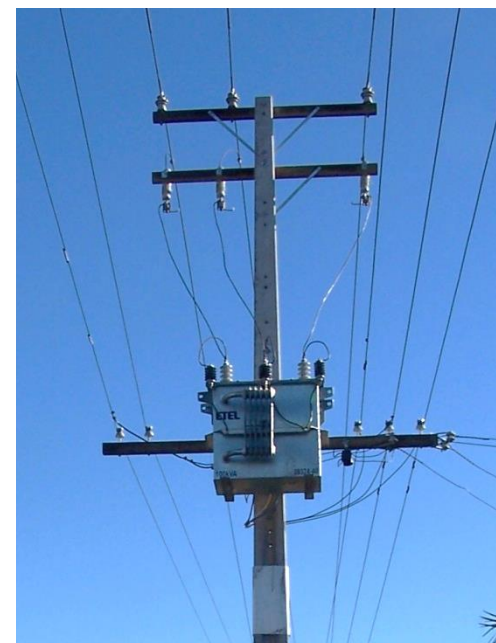
Figure 19.1: 100kVA pole mounted transformer
