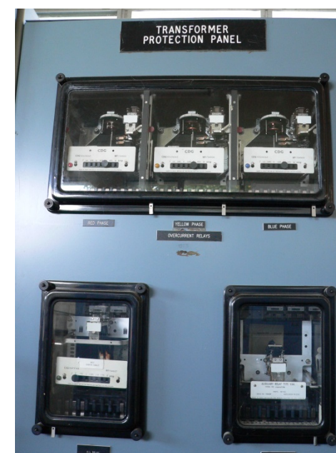
Figure 21.3: Electromechanical relays providing transformer protection
