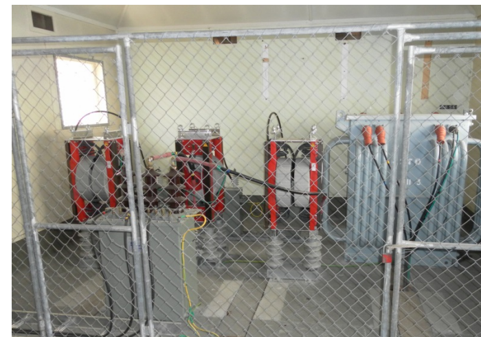
Figure 18.16: Load control injection plant
