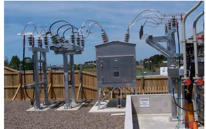
Figure 21.8: Typical outdoor 33kV switchgear bay
