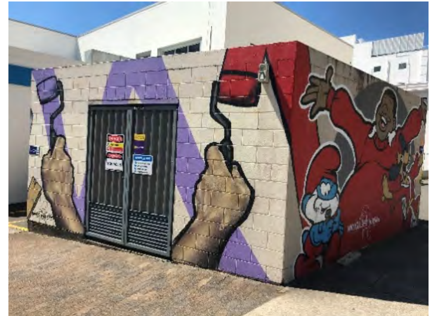
Figure 22.6: Concrete block distribution substation
