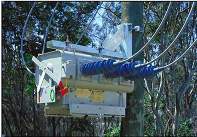
Figure 23.12: A pole-mounted sectionaliser
