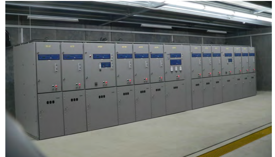
Figure 21.4: 11kV indoor switchboard at Main St, Palmerston North
