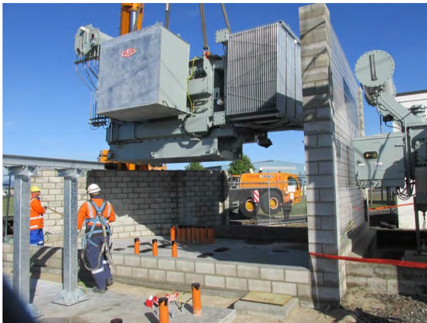
Figure 21.1: Power transformer installation at Waharoa
