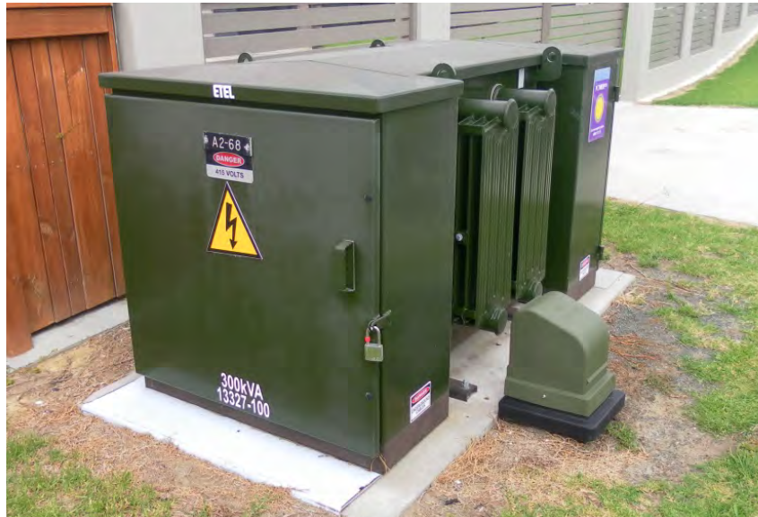
Figure 22.5: 300 kVA ground-mounted transformer
