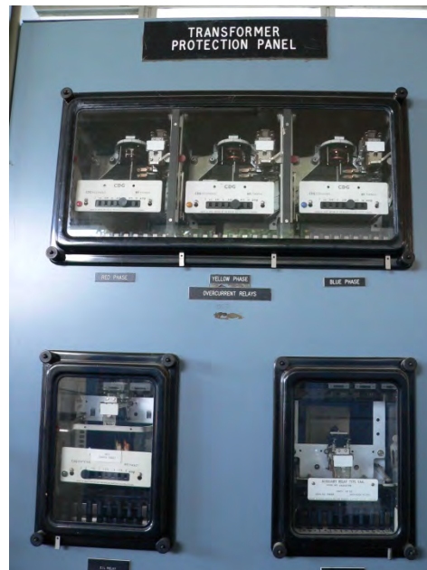
Figure 24.3: Electromechanical relays providing transformer protection
