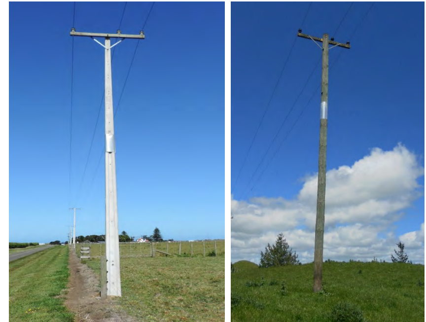
Figure 18.1: A modern pre-stressed concrete pole and a rural softwood pole
