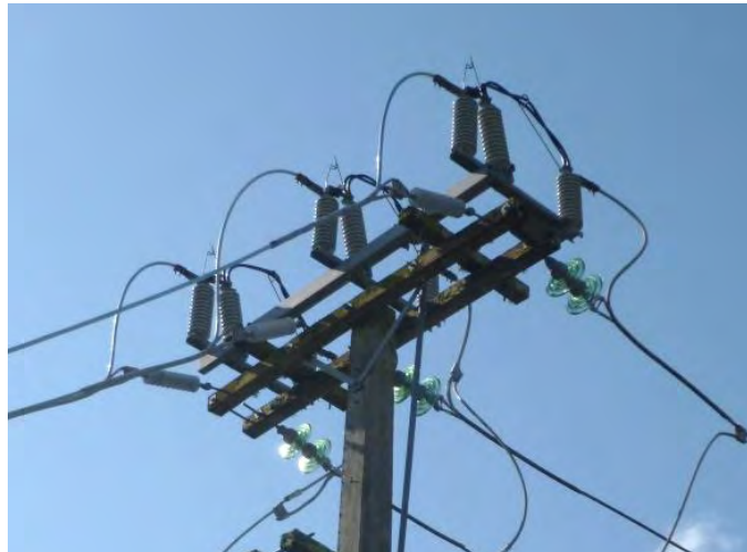
Figure 23.9: Air break switch (ABS)
