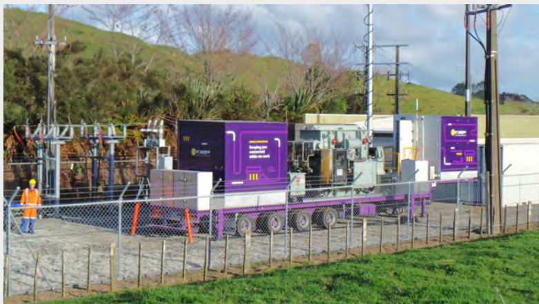
The mobile substation setup at Douglas zone substation.
