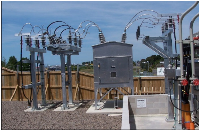
Figure 17.8: Typical outdoor 33kV switchgear bay
