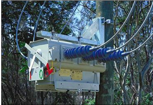
Figure 19.52: A pole-mounted sectionaliser
