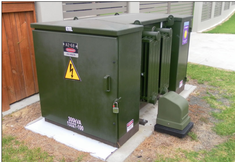
Figure 18.5: 300kVA ground-mounted transformer
