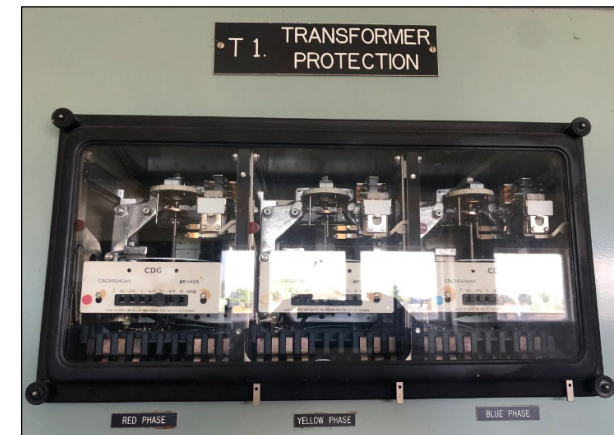
Figure 20.4: Electromechanical relays providing transformer protection
