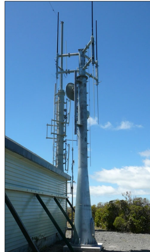
Figure 20.3: Communications mast with associated radio antennae
