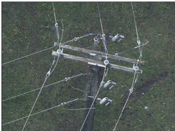
Figure 19.5: Pole-mounted drop out fuse
