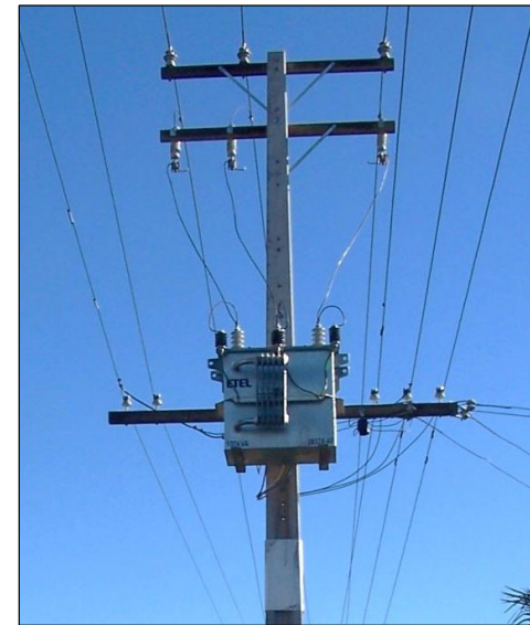
Figure 18.1: 100kVA pole-mounted transformer
