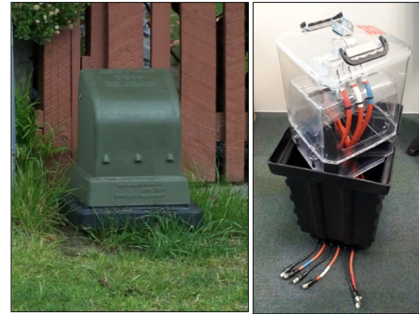
Figure 7.17: Example of organic adaptation. Standard LV pillars (left) are vulnerable to coastal inundation as they are not waterproof. A newer submersible design (shown right).
