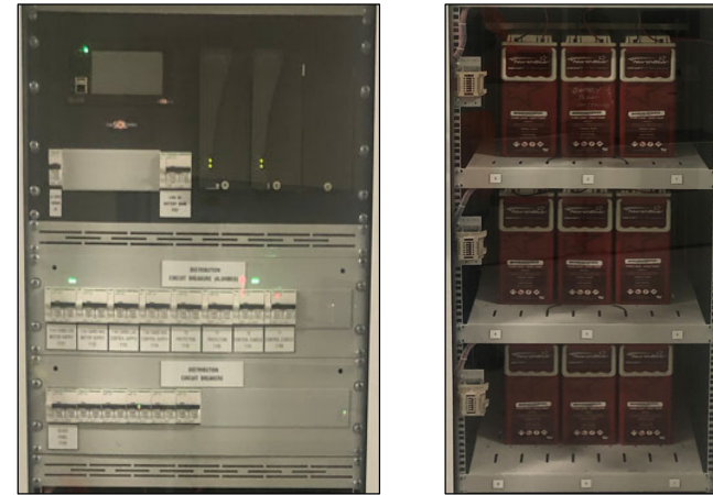
Figure 20.7: DC charger and battery bank
