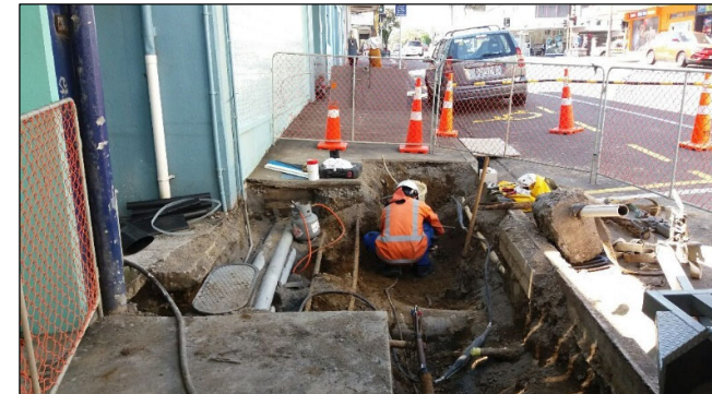
Figure 16.6: Typical urban LV cable environment
