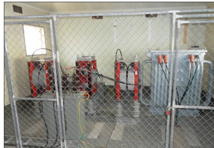
Figure 17.135: Load control injection plant
