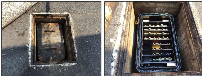
Figure 16.9: Tauranga in-ground pitch-filled LV link pits
