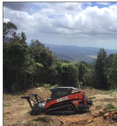
Eco-mulching provides a cost-effective way of creating a corridor around our subtransmission lines.
