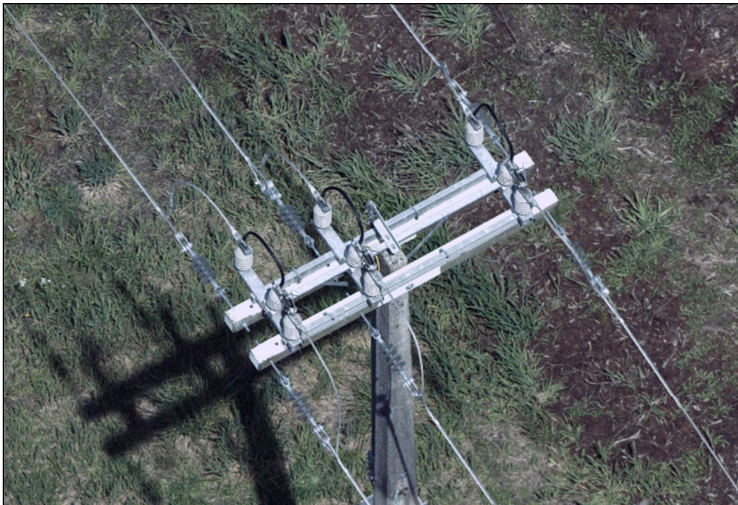
Figure 19.9: Air break switch (ABS)
