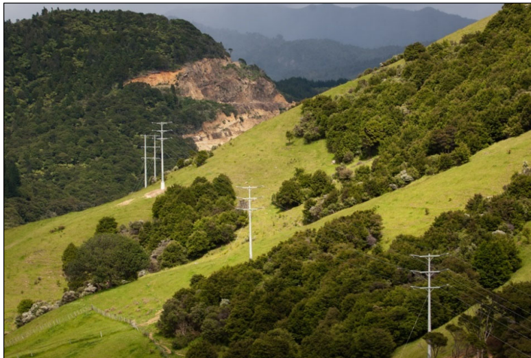
Figure 155.1: 66kV subtransmission overhead line in the Coromandel
