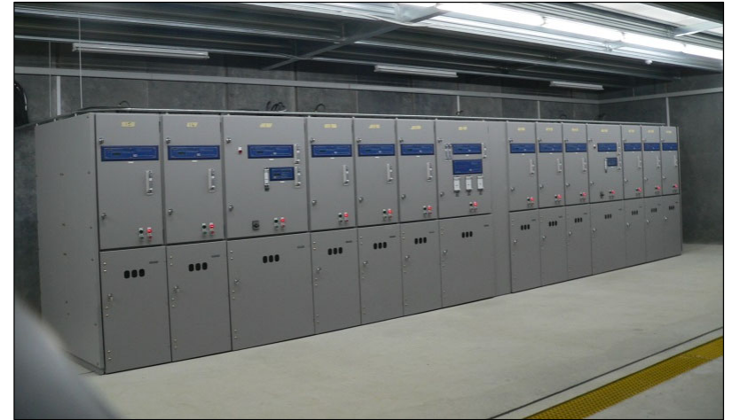
Figure 17.4: 11kV indoor switchboard at Main St, Palmerston North
