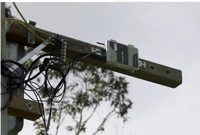
Figure 9 Monitoring device in place
