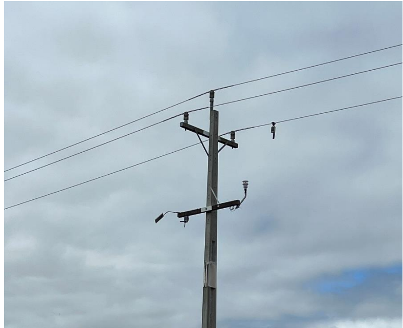
Figure 6 Sensor device and weather station in place
