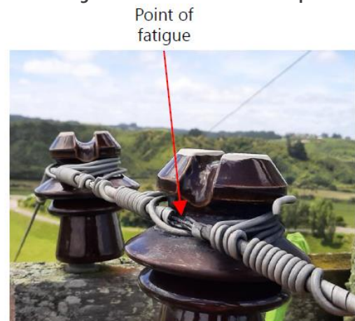
Figure 3 Damage to conductor at attachment point
