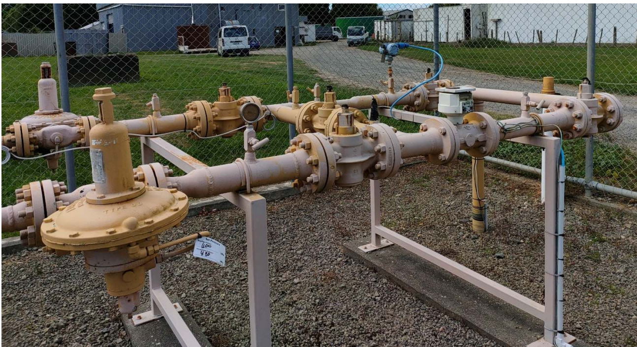
Figure 8 – Levin gate station’s seized, leaking, corroded equipment
