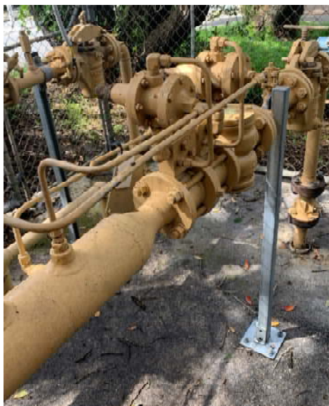
Figure 6 – Chaytor St DRS showing outdated over pressure shut-off valves
